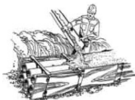
5) The pipes are cast in concrete and sometimes vibrated for good flow.
