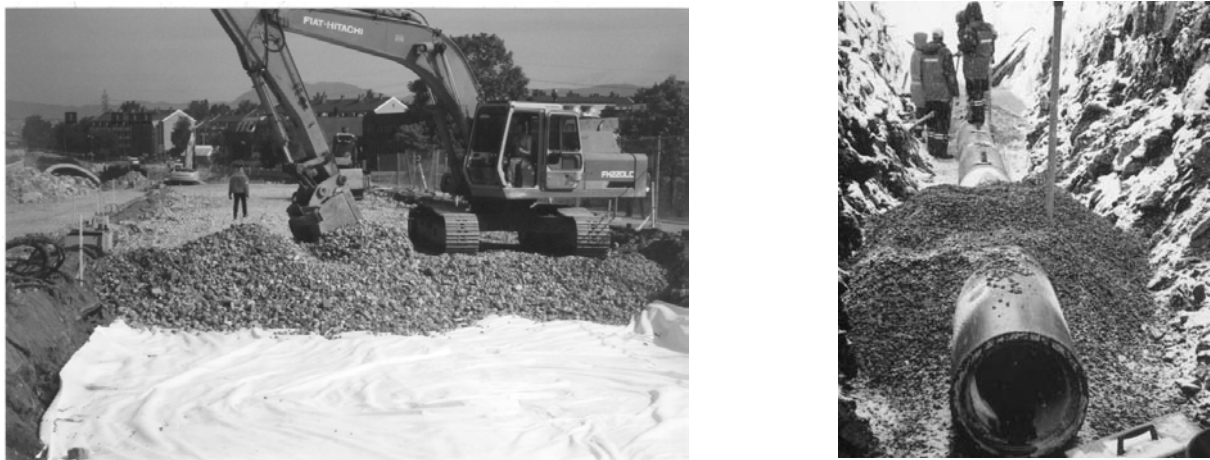
Figure 1 Left: RCA as sub-base in the Svartdal tunnel in Oslo. Right: Landfill in Asker using RCA as backfill in a 600 m utility trench.
