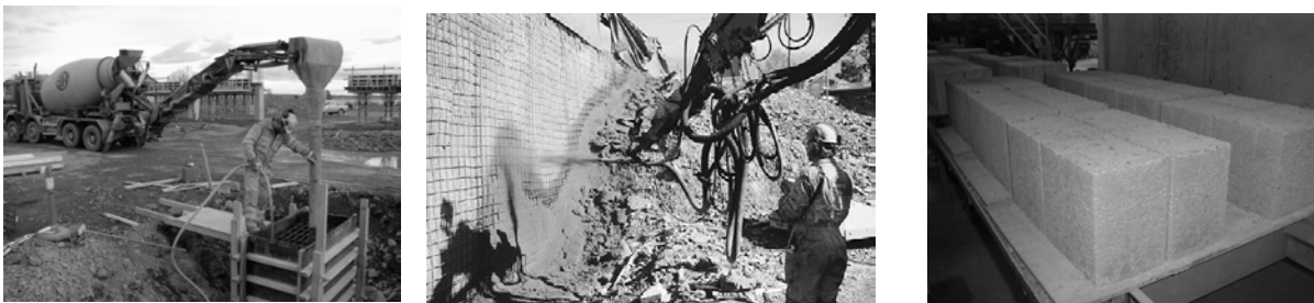
Figure 2 Left: Concrete with RCA in foundations at Fornebu, Oslo. Middel: Shotcrete with RCA in Gaustadbekkdalen, Oslo. Right: Leca's building blocks with 30 % RCA.
