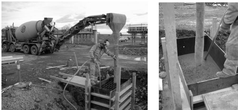
Figure 2 Production of concrete foundation with 20 % replacement of natural aggregates with D_{max} > 8 mm at the Fornebu Building site (Picture: Bente Lillestøl, Veidekke ASA)
