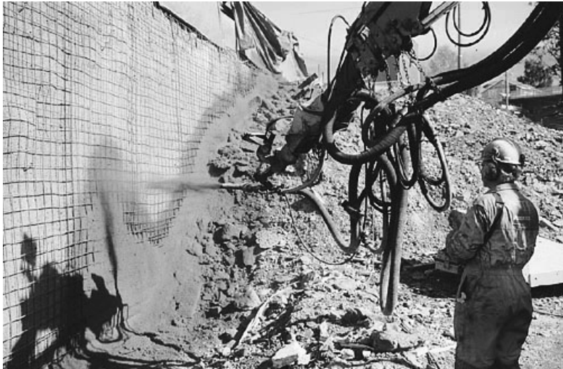
Figure 4 Sprayed concrete with recycled aggregates (0-4 mm) at the Gaustabekk Building site (Picture: Bente Lillestøl, Veidekke ASA)
