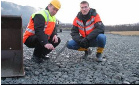
Figure 8: Remaining steel bars may cause a lot of trouble
