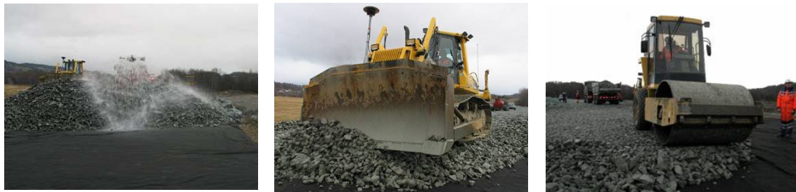
Figure 4. Sprinkling of the crushed concrete materials was recommended before paving and compaction
