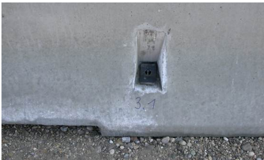
The steel spike is rammed until the weld-on plate is flush with the concrete frame
