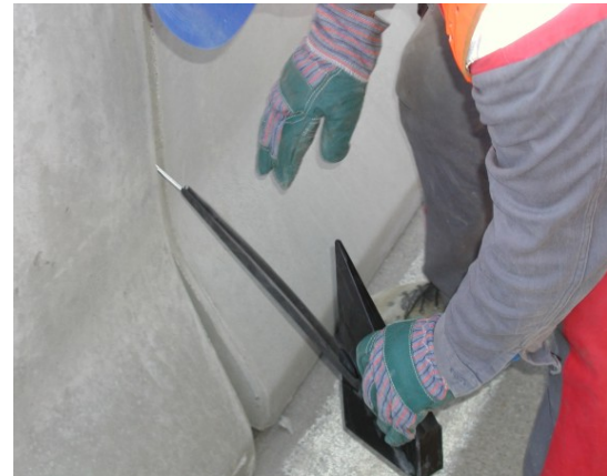
A working stands on either side of the element. Pulling the rubber loop through using a metal hook
