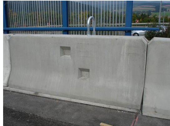
Climbing aid on the lane side
