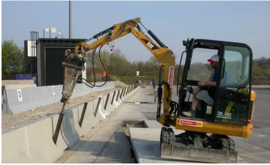
A skid loader with a hydraulic hammer is used to ram the spikes into the subgrade
