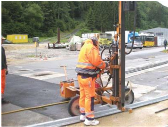
4.7 Lotrechtes ausrichten der Ramme Adjusting the pile driver vertically to the track
