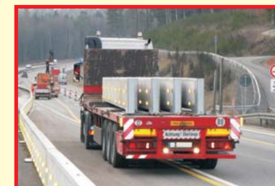
Up to 80 m of ProTec 160 can be loaded on a truck and installed directly from the vehicle.
