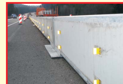
The retractable reflectors are fitted into the concrete in such a way that they recede when touched and are preserved even when a vehicle touches the barrier.
