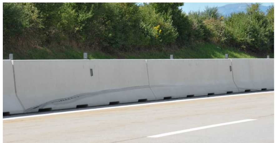
abrasion marks, system not damaged
