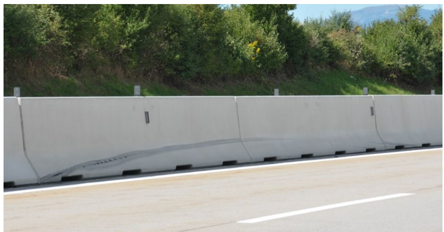
abrasion marks, system not damaged
