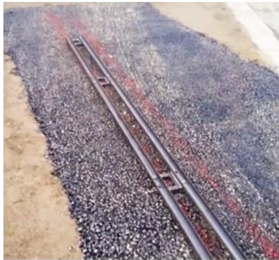
Fig. 8: Positioning of the installation plates by using the template for SMA T2-SMA T4
