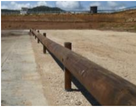
18 cm Round log, 4m length reinforced with a G profile steel on the back.
