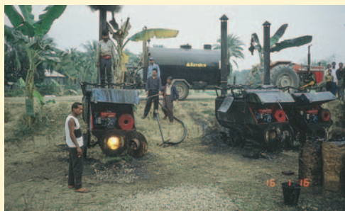
Cutting back to improve the viscosity and binder properties is possible, even under «primitive» conditions. (Bangladesh).
