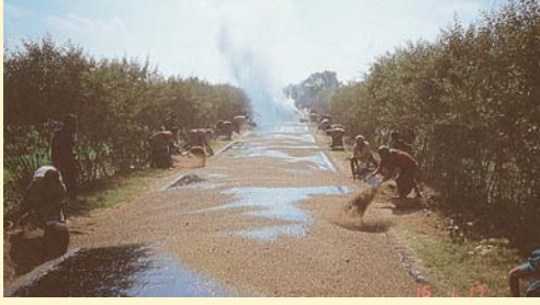
The Otta Seal aggregate was applied by labour based methods, by pre-stockpiling the hand crushed aggregate. A 100 metre long section, 3,7 metres wide was covered by aggregate after 7 minutes time, and the section was opened to traffic. (Bangladesh).
