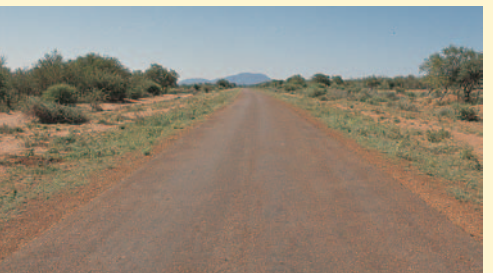
Overview of the same road (Single Otta Seal) after being in service for more than 8 years. (Botswana).
