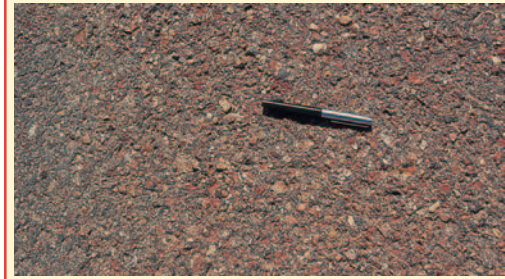
Close-up of the previous photo showing a Single Otta Seal. Note that some of the weak aggregate has been crushed down by traffic, but during the early stage after construction the binder has absorbed the crushed aggregate and a dense water-proof surfacing has been formed. (Botswana).
