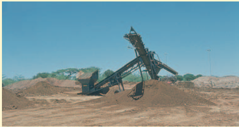
“As dug material” which in many cases only requires screening of oversize materials, can successfully be used in Otta Seals. (Kenya).
