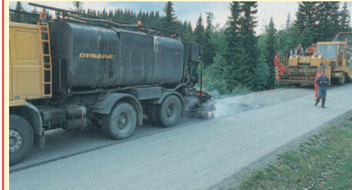
Otta Seals have been and is still extensively used in Norway. (Norway).
