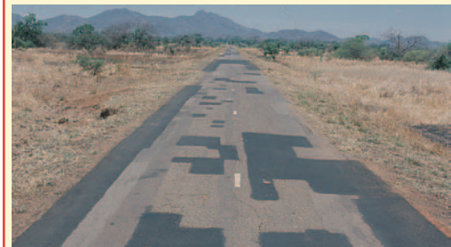
On pavements that have deteriorated badly, an Otta Seal, because of its durability (high bitumen content and low viscosity binders which make the Otta Seal very flexible) is well suited as a reseal. (Malawi).
