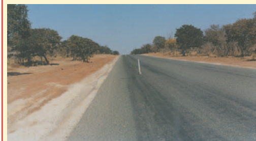
The Otta Seal should preferably be equally exposed to traffic over the entire sealed area as this will enhance an uniform appearance. This can be achieved by the use of traffic cones to direct the traffic in to areas that need trafficking. (Botswana).
