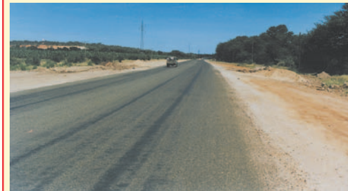
After a period of 8 - 10 weeks (traffic dependent), the Otta Seal beds down to produce the appearance of an asphaltic concrete premix. (Botswana).
