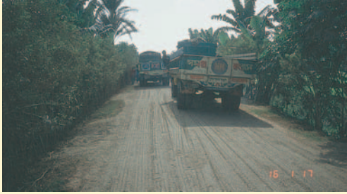
In the absence of pneumatic tired rollers, rolling of the Otta Seal can be done by loaded trucks following a pre-determined pattern of rolling. (Bangladesh).
