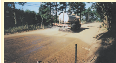
Light watering of the broomed base before spraying the binder will enhance the bond between the base and the Otta Seal. (South Africa).
