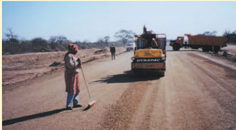
One pass with a static tandem steel roller will improve the embedment of the larger aggregate.
