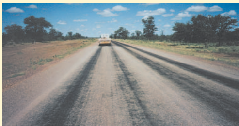
An Otta Seal will for the first few months after opening to traffic exhibit a rich bitumen appearance, which initially appears non-uniform and inferior compared to the conventional Chip Seal. (Botswana).
