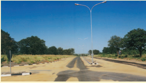
The sand blown off by traffic should be broomed back into the exposed areas until full embedment is achieved. (Botswana).
