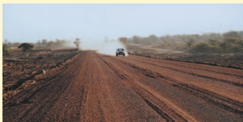
A too excessive aggregate application. (Botswana).
