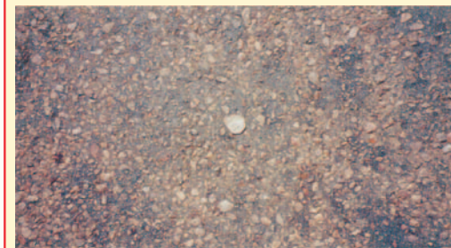
Close up of the Single Otta Seal above. Note the close surface texture, making an impermeable surfacing. (South Africa).
