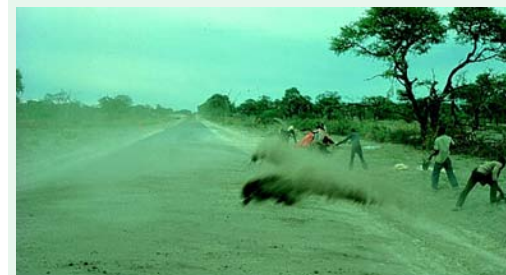
The aggregate requirements for sand cover seal are very relaxed. Kalahari sand directly from the road reserve area can be used successfully for this purpose (Sehitwa - Tsau road).
