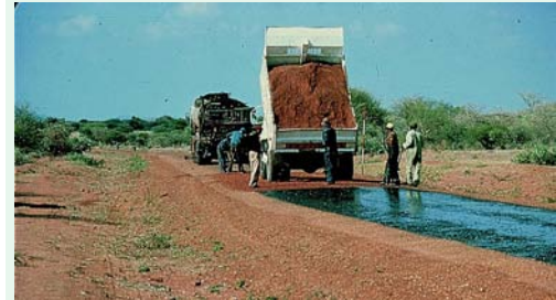
Labour based methods were used by applying the Otta Seal aggregate by hand.
