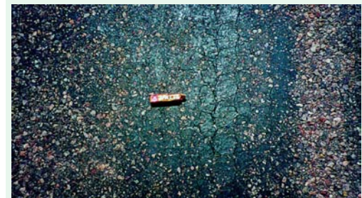
Bitumen being pressed up in-between the aggregate particles, sparsely distributed in the wheel paths, indicates that the bitumen/aggregate ratio is correct. The photograph shows excess of bitumen due to over-application of the binder.
