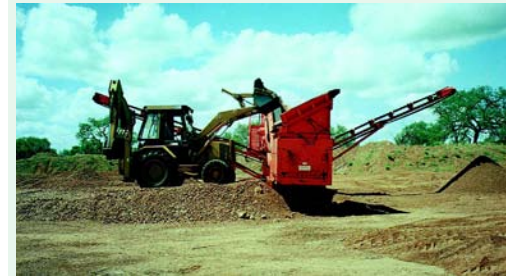
The wide grading envelope allowed for the Otta Seal maximises the use of natural gravel (as-dug material), which in many cases requires only screening of oversize materials by use of a power screen (Mahalapye – Machaneng road).
