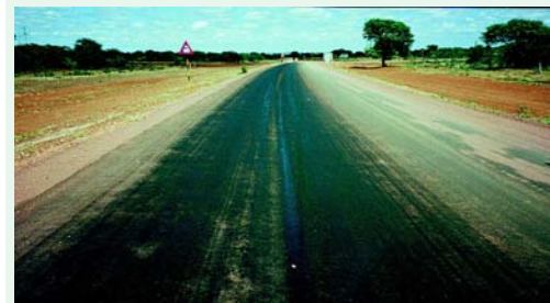
Some bleeding in localised areas and in the wheel paths form a normal part of the curing process. Severe bleeding can be rectified by sand or additional aggregate rolled into the bleeding areas.
