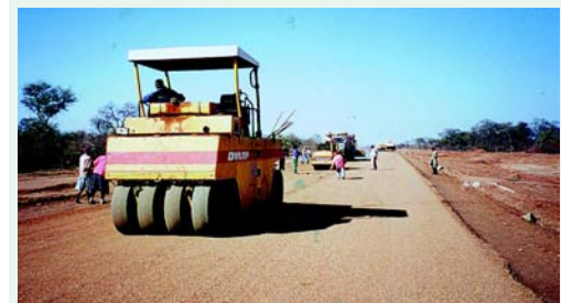
Extensive rolling with pneumatic rollers is essential to achieve a good result.
