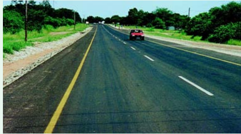
A bituminous surfacing provides good riding quality and protects the base course layer. Single Otta Seal + sand cover seal using Kalahari sand (Kasane – Ngoma road).
