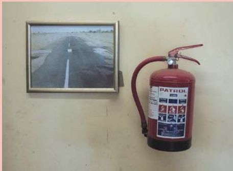
Fire extinguishers shall be placed in clearly visible places with unrestricted access.
