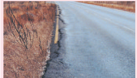
Shoving due to unstable base course layer.
