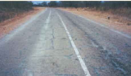
Block cracks resulting from stabilised base. They have been well sealed to prevent water ingress.
