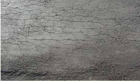
Crocodile cracking and associated shoving.
