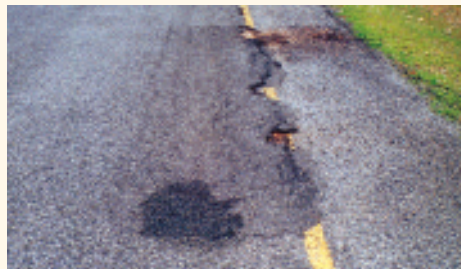
Large patch but poorly executed resulting in failure.
