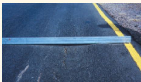
Pavement distress, shown as excessive rutting.
