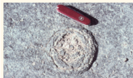
Close up of salt blisters.
