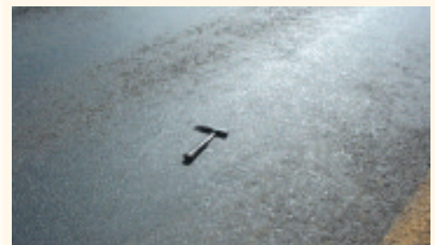
Loss of surface texture as a result of bleeding (degree 5).
