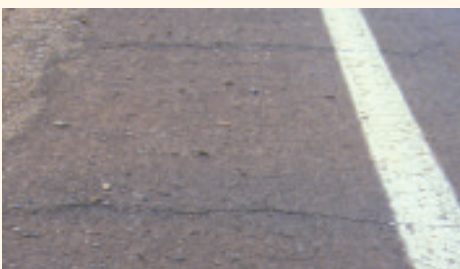
Transverse cracking is very common and is usually caused by temperature-associated distress.
