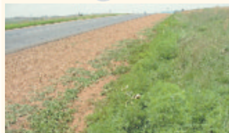
Inadequate maintenance of side drains.
