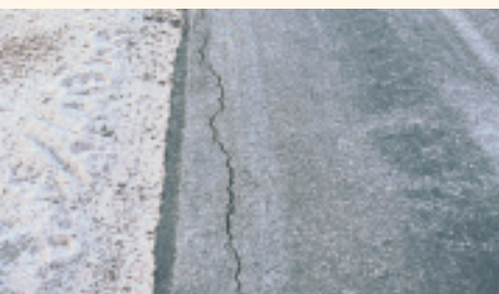
Swelling of subgrades or settlement of embankments may also cause longitudinal cracking. Such cracks are not confined to the wheel paths and are often found near the shoulders of the pavement.
