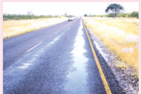
By carrying out visual inspection immediately after rainfall, pavement defects such as rutting/depressions clearly show up.
