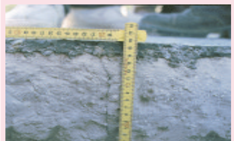
A photograph like this will help in recalling details, such as the crack through the base layer.
