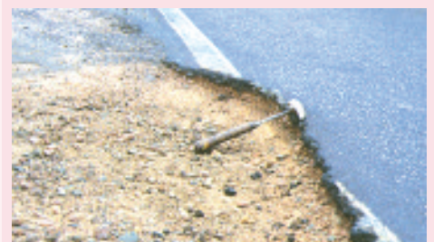
Excessive shoulder drop off.
