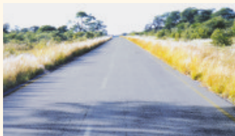
Grass and bushes should not be allowed to grow close to the surfaced area, as this will have a negative influence on the pavement performance.
