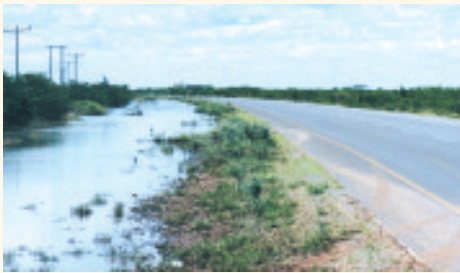
Adequate drainage of the pavement layers and subgrade is essential for good pavement performance.
