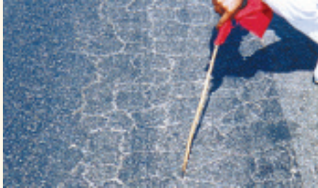
The presence of pumping is a sign of serious deficiencies in the base layer and normally signals the onset of rapid deterioration.
