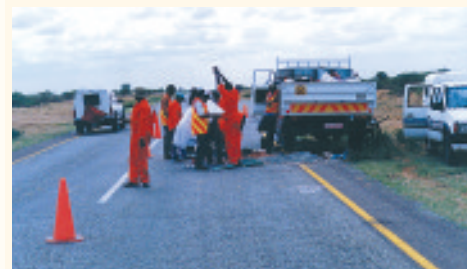
Field testing and sampling is costly and should be carefully planned and executed.
