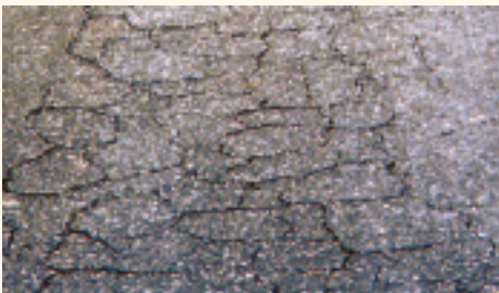
Typical map cracking.
