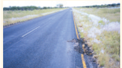
Localised structural problem.
