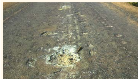
Salt damage to road surfacing.
