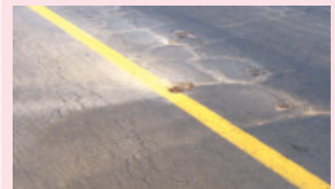
Degree 5 pumping resulting in potholes.
