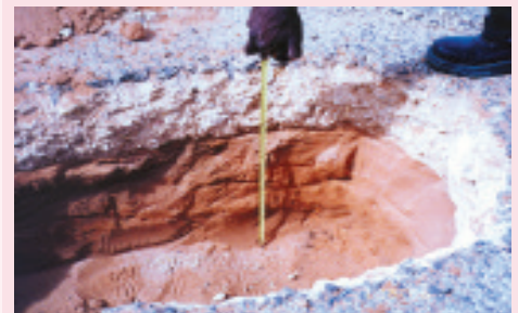
A photograph of the wall of the test pit (including a scale) can assist with recalling details regarding the pavement during later evaluation of the data. Identification of the location and details of the pit should be included in the photograph.
