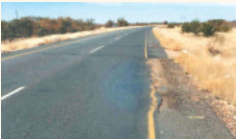
Typical sign of pavement distress in the form of outer wheel path failures.
