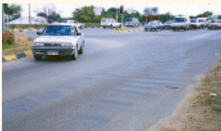
Unstable premix causes shoving.
