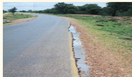
Water ponding at the edge of the surfacing will weaken the pavement structure.
