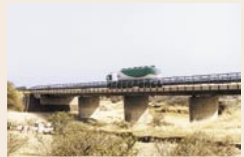
Heavy axle loads impose a different impact on a bridge than on a road pavement structure.
