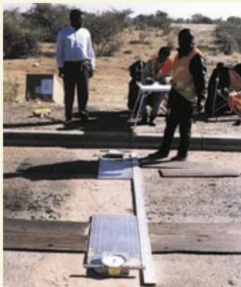
Fine dry sand shall be used to even out irregularities under the platform for the mobile weigh bridges. This will prevent sharp stones to punch into the platform.
