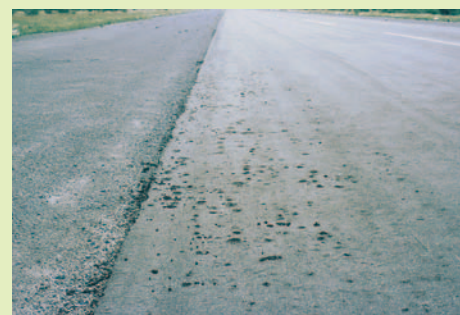
Salt damage to shoulders. Damage will normally start at the shoulders and progress to the centre of the carriageway. This is due to high evaporation and less traffic at the shoulders.
