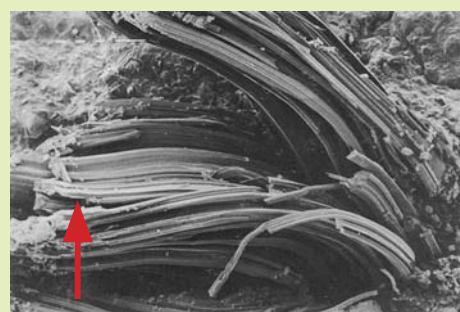
Microscopic sized salt whiskers breaking through road surfacing. This type of crystal causes maximum damage due to high pressures.
