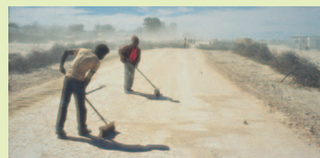
Brooming was used successfully on parts of Sehitwa-Tsau, Tsau-Gumare and Tsabong-Makopong roads.
