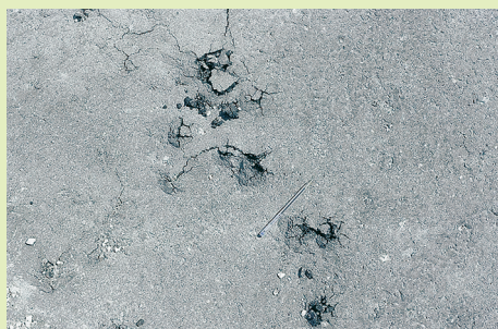
Salt damage is often observed within days after priming or up to 2-3 days after surfacing. Tsabong - Makopong road.
