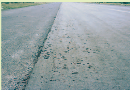
Domed cape seal surfacing due to salt attack Sua Pan Airstrip.
