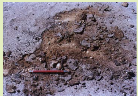
Powdered cutback prime and top of base course due to salt attack. Nata - Maun road.
