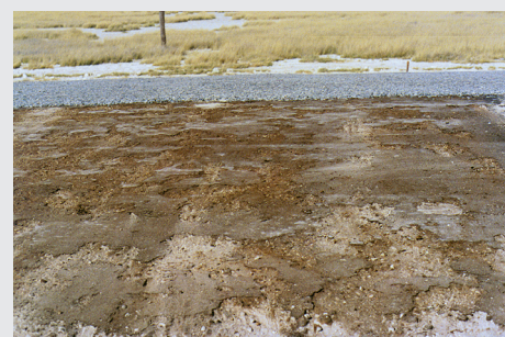
A base course layer with high salt content. The prime has been exposed too long before the surfacing is applied and deterioration of the prime is the result.
