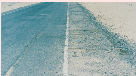
Shoulder deterioration can also be caused by other factors such as insufficient binder spray rate.
