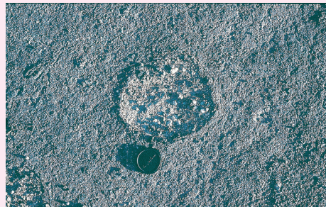
- resulting in an exposed base.
