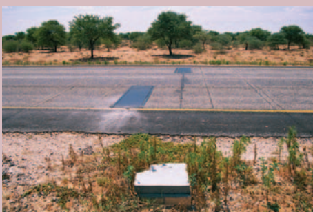
A speed, axle and traffic flow data collection station with a lockable counting equipment box.
