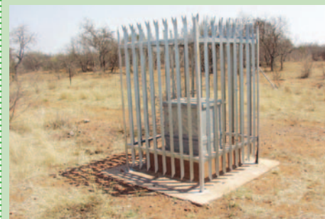
A security fence for traffic counting equipment.
