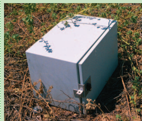
A roadside box or cabinet for storage of a traffic counter.
