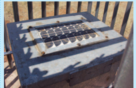
Automatic counting station secured and operated by solar power.
