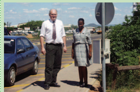
Counting equipment fixed to a traffic signpost.
