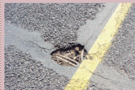
A damaged road surface exposing induction cables is prone to damage.
