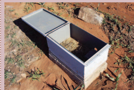
Lack of proper maintenance can lead to some stations being rendered un-operational and loss of important traffic data.
