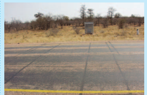
Typical installation of inductive loops.
