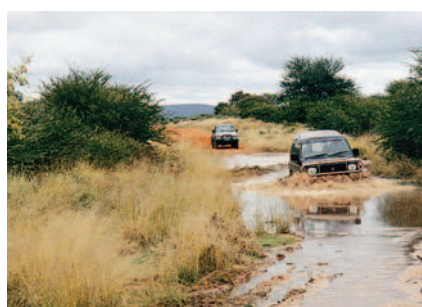
Short sections of road in poor condition can benefit significantly from spot improvement works.
