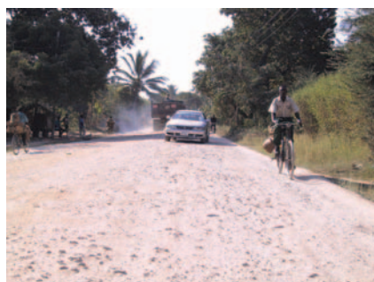
Due to loss of fines, gravel roads often become very rough which make driving conditions hazardous and, in addition to severe driver discomfort, impose very high vehicle operating costs.
