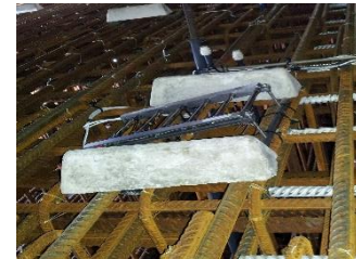
[Corrosion monitoring sensor] [33]
