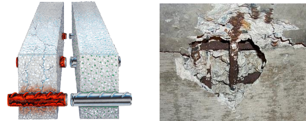
[Rebar corrosion of reinforced concrete structures] [31][32]
